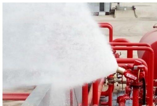
Foam System Package Smart Refinery-Tarjun
